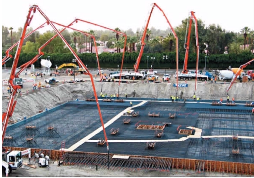
Concrete trucks poured more than 600 loads of concrete, using six pumps to evenly distribute the concrete to create the foundation of the Walter and Leonore Annenberg Pavilion.
